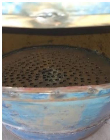
Figure 3. Iron Plate In the Combustion Chamber
