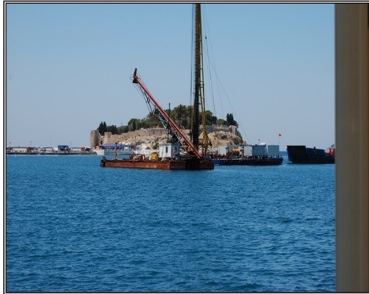
Figure 3. Floating concrete wharfs constructed to increase the Kusadasi ports capacity (2011)
